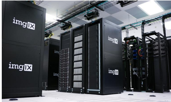
Figure 1: Server room. Image courtesy of imgix on Unsplash
